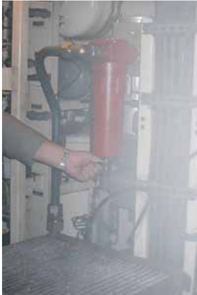
Oil mist from a downstream filter, which has by-passed the dryer and oil filter and would otherwise pass into the braking system or other application; these require clean, dry air for reliable operation.
