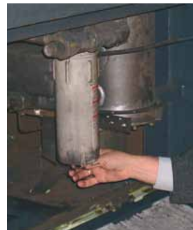
Oil removed from a downstream coalescing filter fitted after a desiccant air dryer (adsorption dryer)
